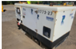
Pramac 33kVA Skid Mounted Diesel Generator - choice
